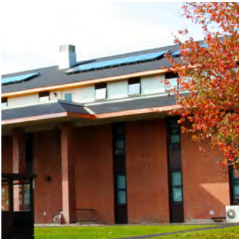
Solar Hot Water Roof Panels
